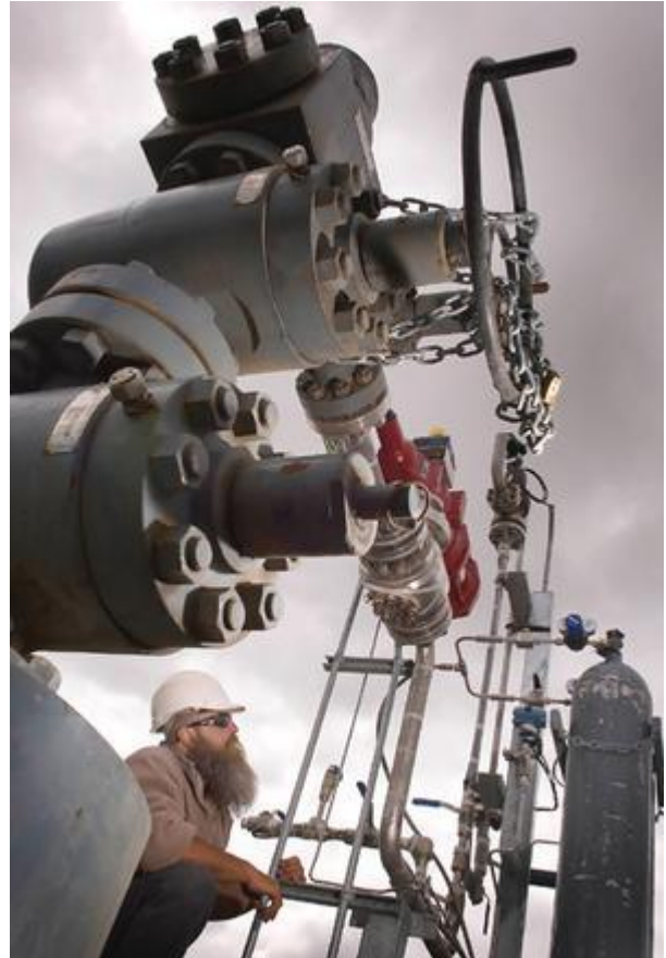
All geared up to send 100,000 tonnes of carbon dioxide underground near Warrnambool.
